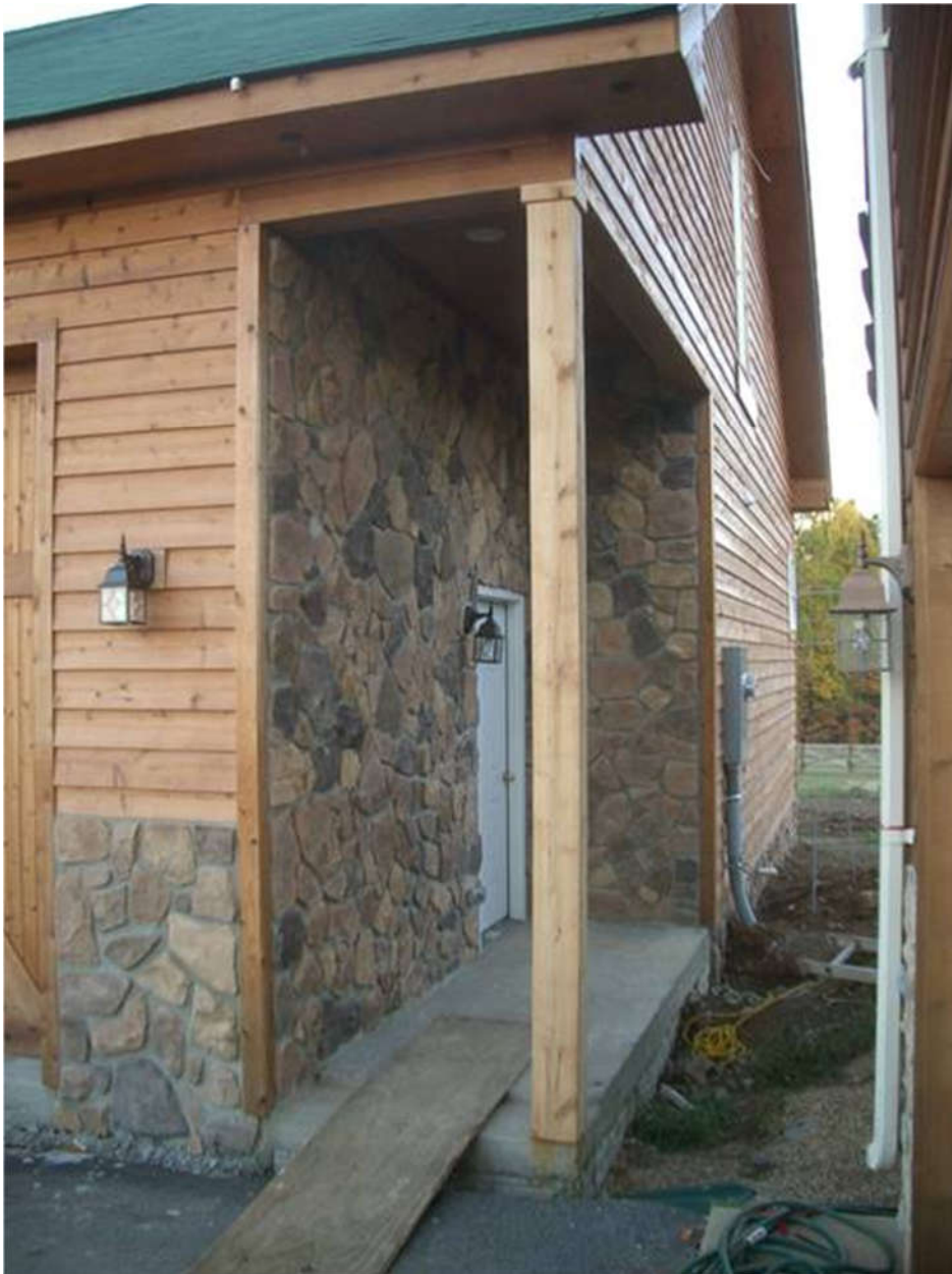
Construction photo showing the breezeway cutout I designed into the modified plans to allow the building to be within 4' of the house, and thereby sidestepping county regulations. You can see how close the building really is to the house.
